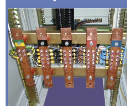
500 Amp. Power Bars
